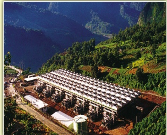
FIGURE 6: Geothermal power plant at Zunil, Guatemala.
