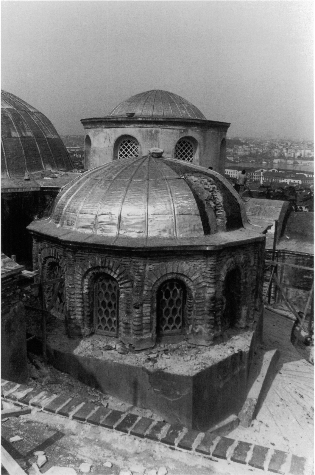
8 Zeyrek Camii, view from South Building, looking north, showing roofing in progress and eastern dome of Middle Building during repair, 1998
