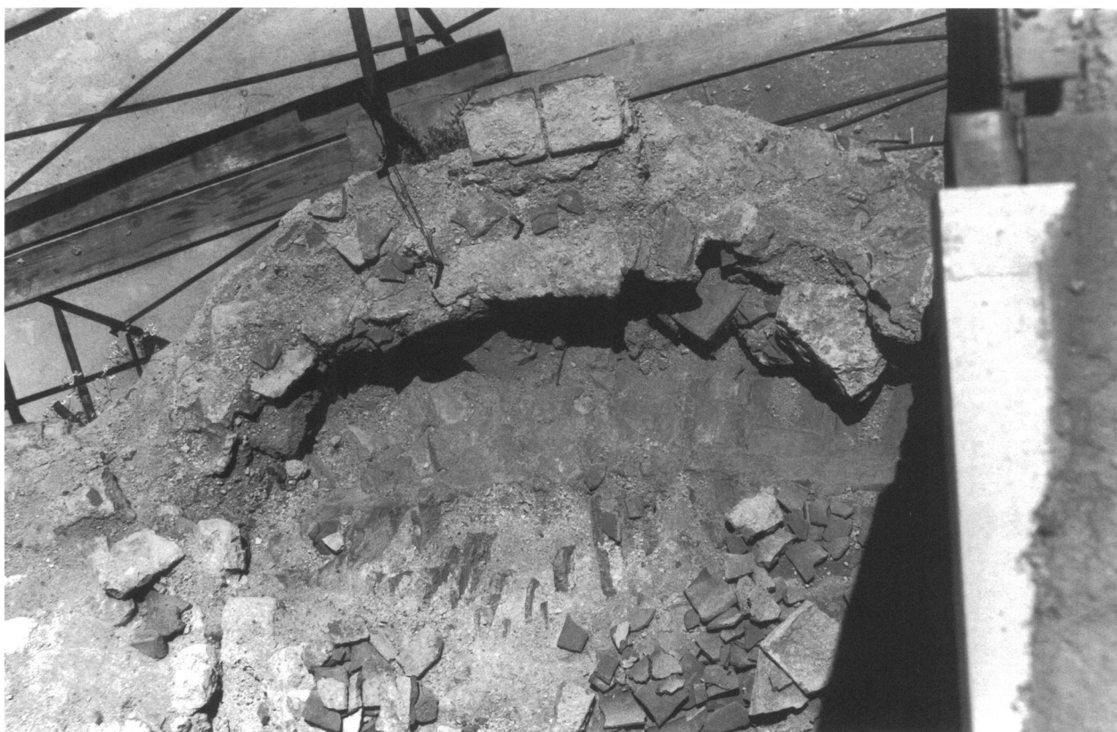
10 Zeyrek Camii, North Building, vaulting of the prothesis, showing Byzantine roofing tiles above the conch, 1998
