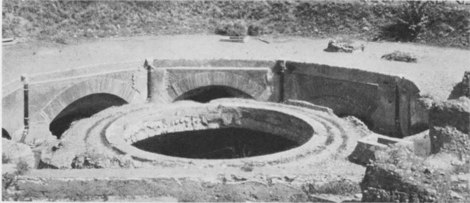
416 Construction of the cupola and openings for lighting of the octagonal hall.
