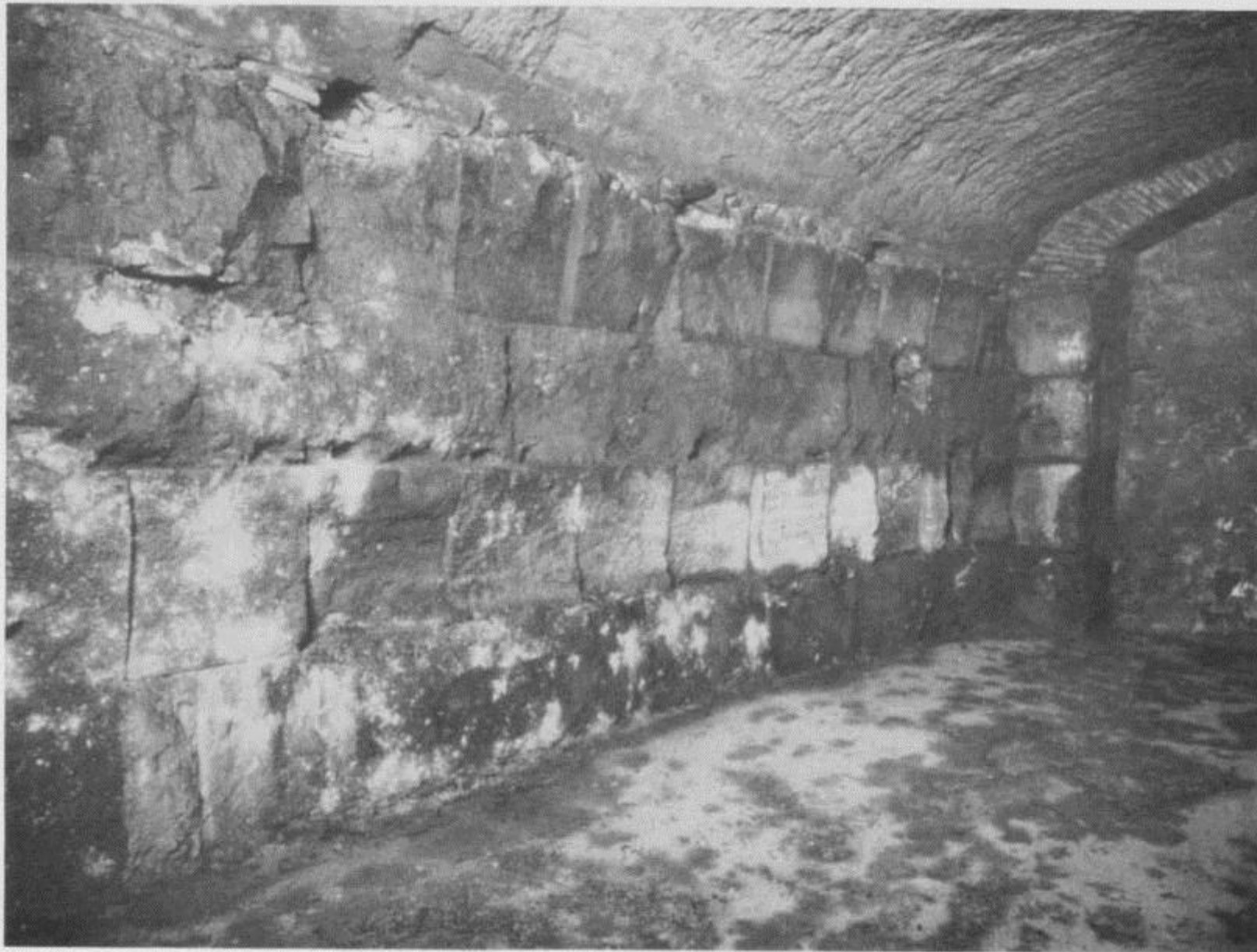
1220 Tufa foundations for the steps which led up to the Temple of Venus Victrix, seen in the Palazzo Pio-Righetti. Rip X C/3290
