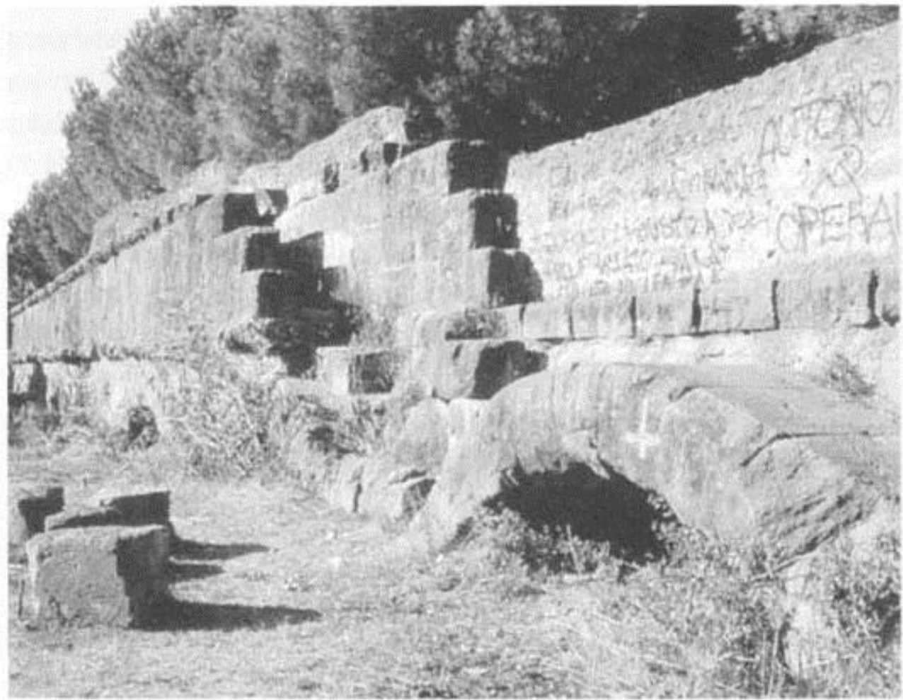
Fig. 8.3: The channel and arcade of the Aqua Marcia at Romavecchia. The channel of the Aqua Tepula partially survives on top (Photo: author).
