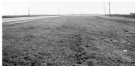
Typical Roadway with Roadside Hazard Rating Equal to 1.
