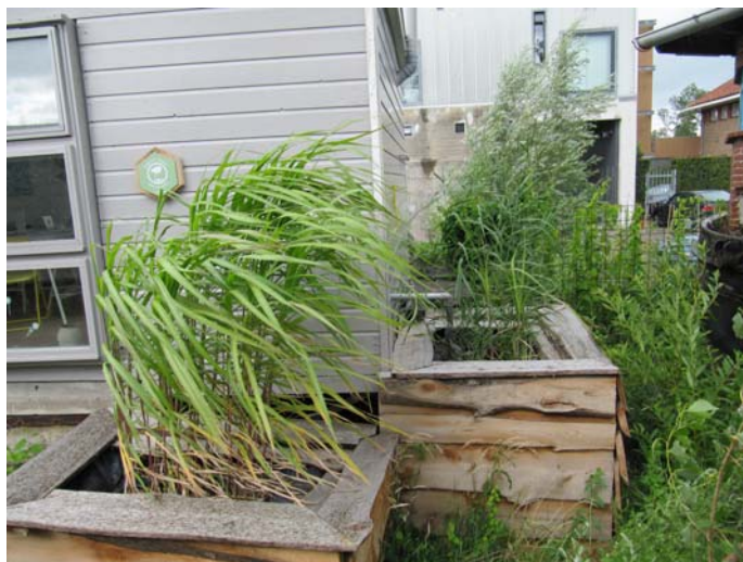
Fig. 2. Grey water treatment in individual low-tech biofilters, consisting of two IBC containers filled with layers of gravel and coarse and fine sand, planted with reeds.
